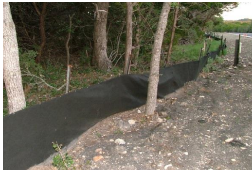
Temporary Silt Fence
